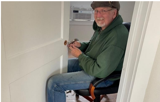
Above: Donnie Yost, Jr. of Elmo showed up to assist the Community Service Day at the Annex! He is seen here installing door knobs.
